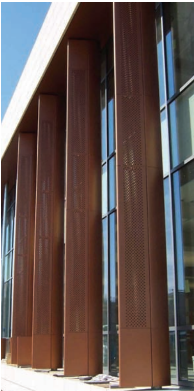
Custom Column Covers Johnson Controls, Glendale, WI Architect: Gensler
